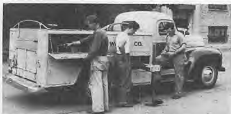
Utility Truck Operating Distribution Valve
